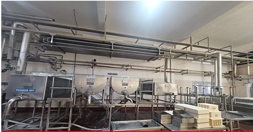
Panner Plant capacity increased from 700LPH to 1200LPH with same energy usage
