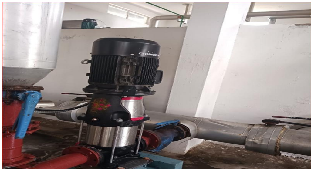
IBT Chilled water Pump
